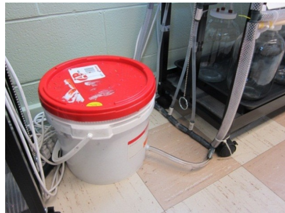
Figure 10: Bucket of activated charcoal to filter out-flow air of any contamination
