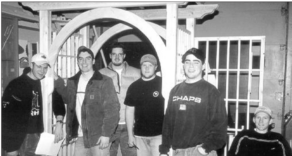
The Wood Construction Techniques Class constructs an Arbor out of cedar that will eventually be placed in the Alumni Gardens along with fences. When the project is completed four such Arbors will be built as entrances to various sections of the garden. (L to R) Andrew Hayes, Gabriel McLaughlin, Jeffrey MacDonald, Peter Kiersted, David MacKenzie, and Gordie Campbell.
