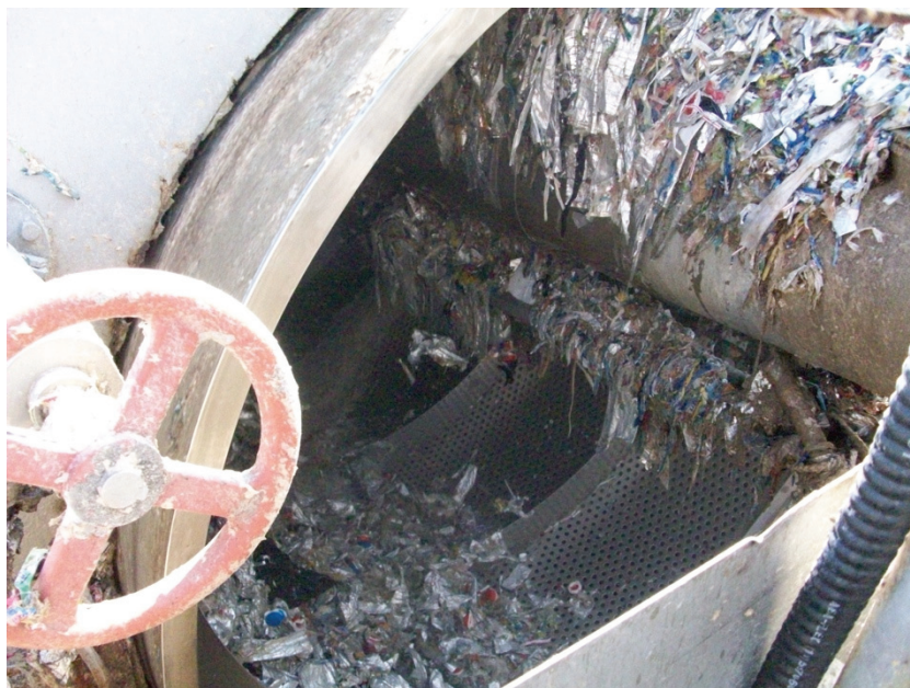
Figure 4.5: Detrashing screens downstream of the hydropulper used to recover process water in Piracicaba, Brazil.
