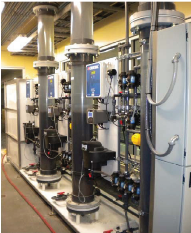
Figure 3.3 Photo of pilot plant filtration skid.
