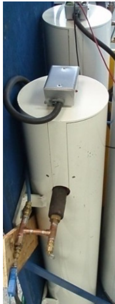
Figure 56 The electrical heaters.
