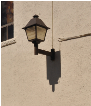
Vivian Lane. Lights attached onto wall.
