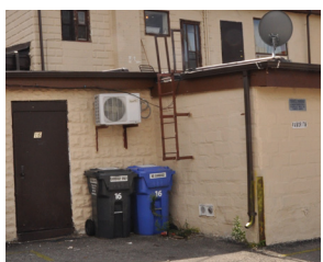
Diplock Lane. Image showing mechanical units, egress ladders and eaves troughs attached to existing building.
