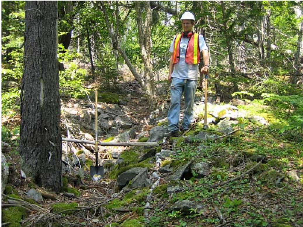
Figure 6.15 Subsidence almost perpendicularly intersecting line#3 at stations between 12 and 20: Matthew Halliday stood there for a reference of the size and depth of this subsidence
