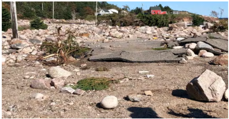
Destruction to New Heaven Road, Neil's Harbour, after extreme storm surges from Hurricane Fiona, 2022 (Ayers 2022).
