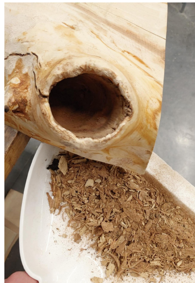
Removing the rotten wood to preserve the remaining wood in the knot
