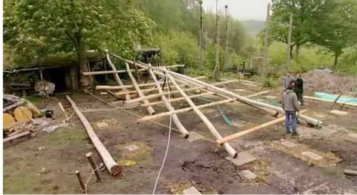
“A” frame bents assembled and stacked on the ground prior to raising the structure with ropes and pulleys. (Mcloud 2003)
