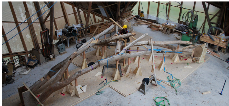
Tree forks being assembled. Notice the large rubber mallet and sledge hammer on the right hand side of the image (Hooke Park 2016).
