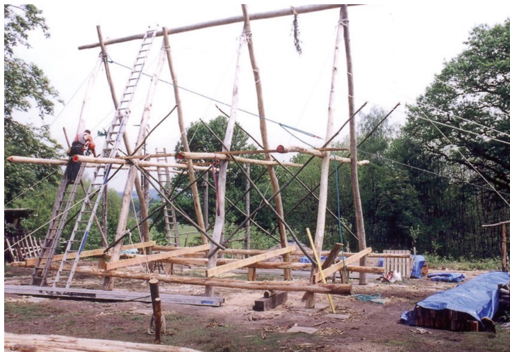
The standing frames. Guidelines and temporary bracing are holding the structure in place. (Law 2022)
