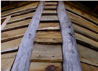
Wood siding over stud wall behind and scribe fit around grown form posts (Mcloud 2003).
