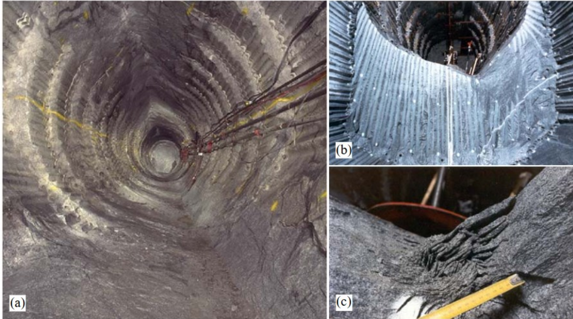
Figure 2-8: MBE tunnel: a) final v-shaped notches; b) cross section of notch in tunnel invert; c) notch-tip in tunnel invert (Read, 2004)
