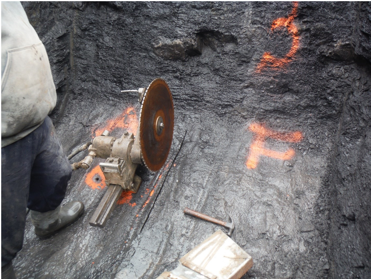
Figure 50: Test pit 3 where the 26-inch diameter saw was installed and the slot was successfully cut. This saw and mounting hardware could be pulled easily out of the ground after vibrations due to cutting.
