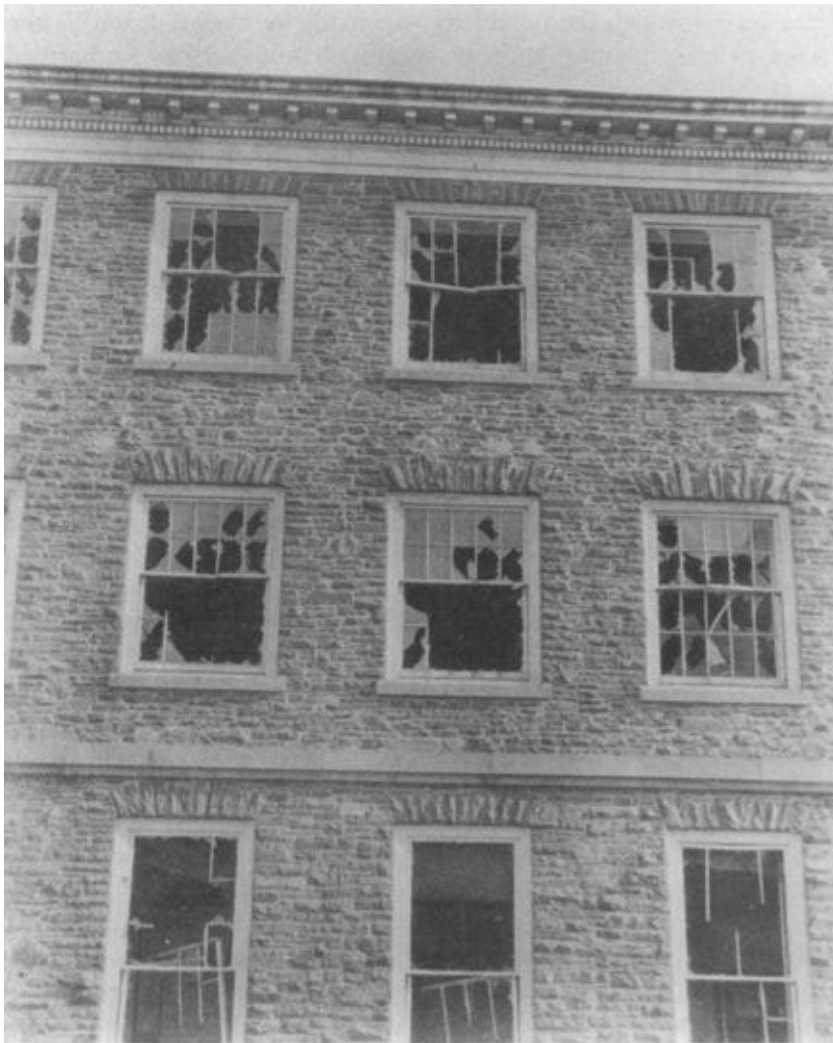
Damage to windows on the east end of the Science Building by the 1917 explosion.
