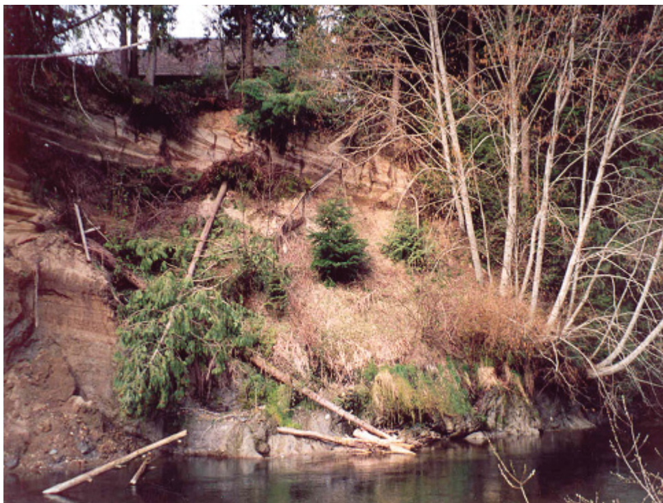
Illustrating coastal slump slide failure (Vancouver Island University 2015)
