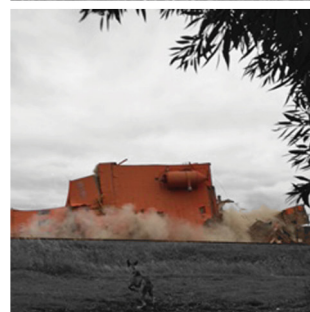
The demolition of Carey's Pioneer Elevator, 2014; photograph by Matt Raffard, from email to author.
