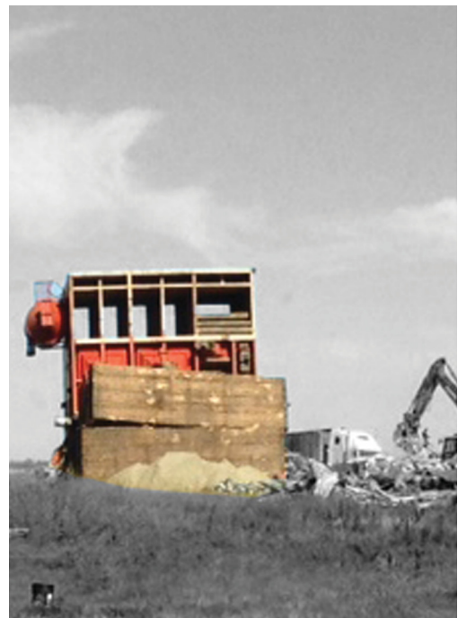
The Carey Pioneer grain elevator fallen to the ground while workers clear the site, 2014; photographs by Anja Eliassen from email to author.
