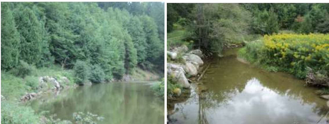
Figure 4.12 Big Head River Watershed restoration projects. Bankside armouring (left) and stream channel restoration (right).
