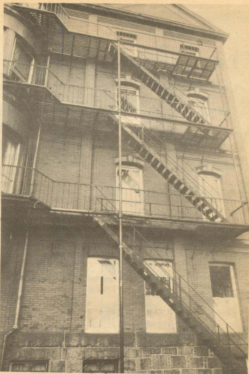
This is the fire escape at the back of the Halifax School for the Blind at University Avenue and South Park. Presumably, in the event of fire, blind schoolkids are supposed to find their way to safety down these stairs. BRAM maintains that facilities at the school are inadequate.
