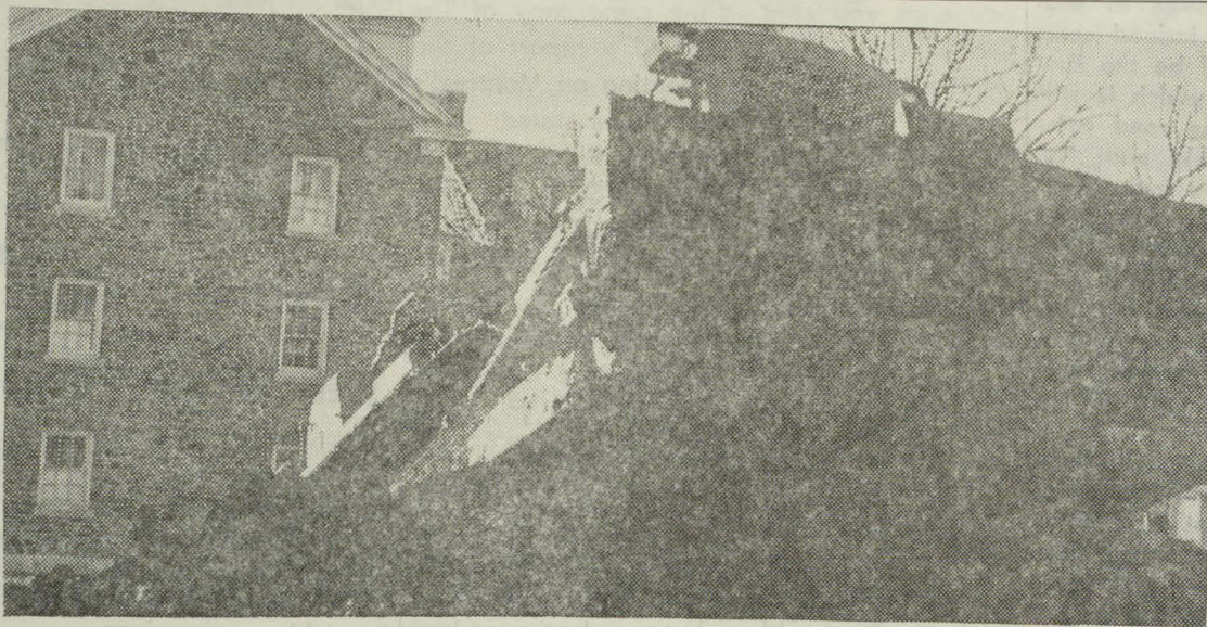
EXPANSION AT KING'S — For the past few weeks, construction crews have been busy excavating the King's College campus prior to building a new women's residence, gymnasium, and dining hall. The women's residence will be partly financed by a Canada Council grant.
