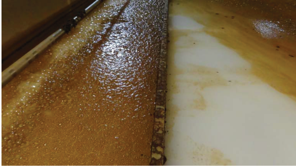
Figure 4.7. Surface of DAF tank showing whitewater, skimmer and sludge blanket.
