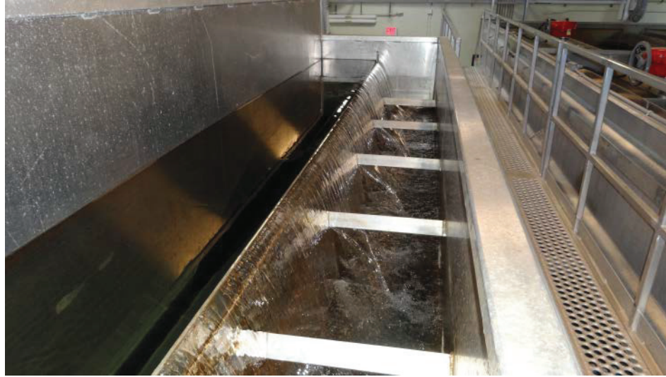
Figure 4.8. DAF tank exit weir overflowing to filter supply pipe.
