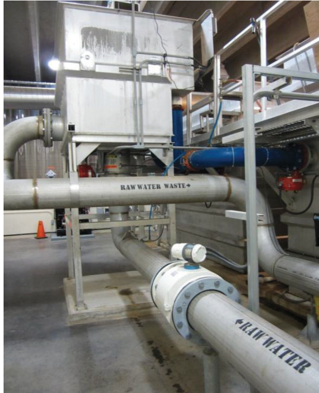
Figure 4.4. Raw water supply pipe leading to flash mixer tank.
