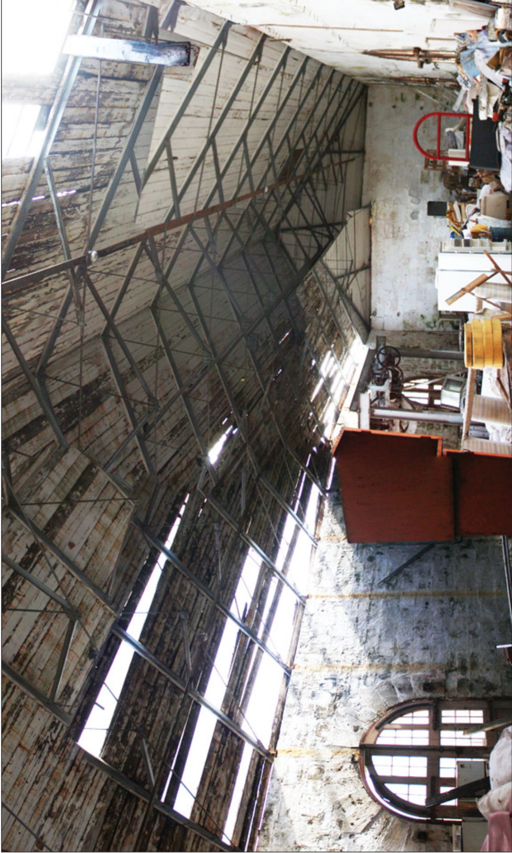
Existing Conditions Photomontage. The South wing of the Storehouse No. 2 has suffered roof damage as a result of recent storms and lack of upkeep.
