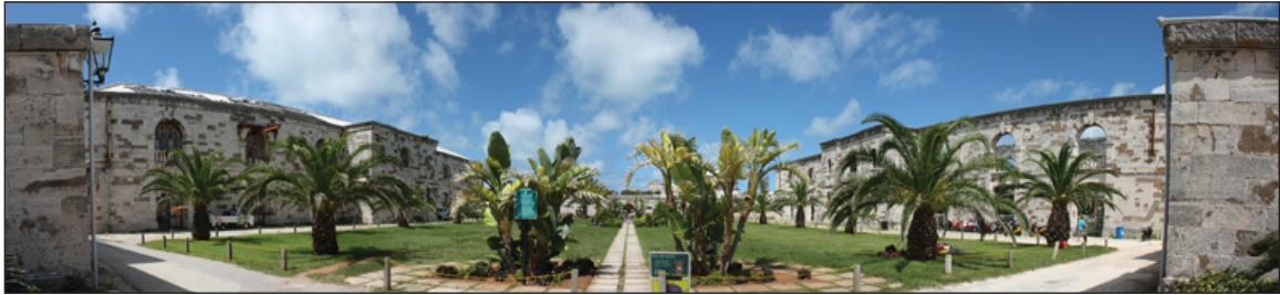
View of the Victualing Yard from the Southern entrance. (Right) Storehouse No. 1 (Left) Storehouse No. 2 both standing in disrepair.
