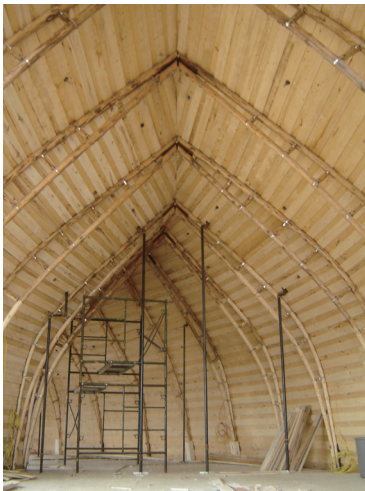
Interior Structure of Pictou Landing Health Centre. Photo by swvander22 From flickr.com.
