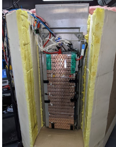
(k) Test unit with battery installed
