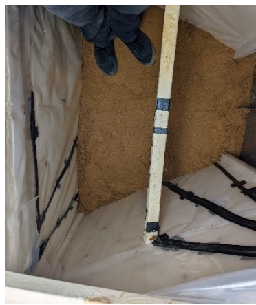
(h): Soil compaction
