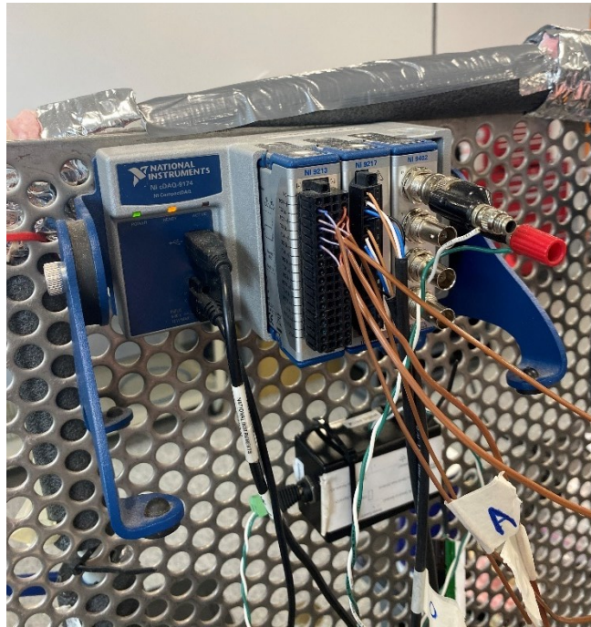
Figure 3.12: Ni-cDAQ-9174 chassis and modules
