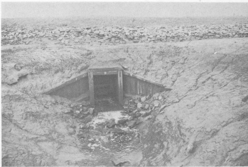
Figure 8 – Seaman Marsh, Cumberland County, N.S. – A typical small sluice structure with a bronze 1\frac{1}{2}' \times 2\frac{1}{2}' gate.
