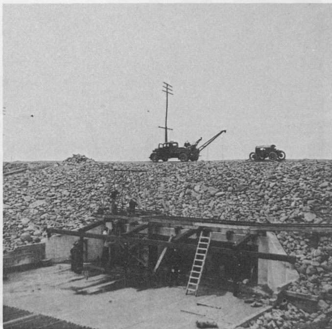
The down stream side of the fresh water control structure through which the Isgonish River has been diverted. The gates, to stop tidal flow, are being installed prior to the damming of the river itself. Trans-Canada Highway traffic will cross over this structure. June 1955.
