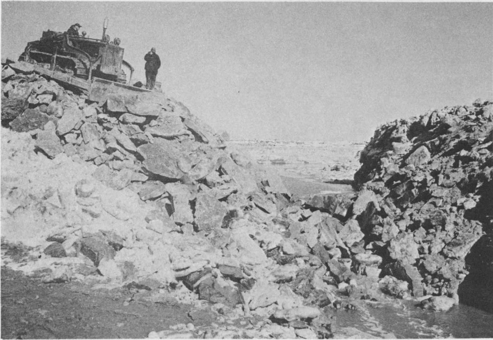
Closure about to be made in the rock fill dam on Palmer's Creek, Dorchester Project near Dorchester, Westmorland Co., N.B. This structure, in combination with the discharge sluice and dyke adjacent to it, does away with the need to reconstruct considerable dyke and several aboiteaux. Future maintenance costs will be reduced as a result and land which would not otherwise be reclaimed is made suitable for production. March 1956. (Photo N.B. 13//41)
