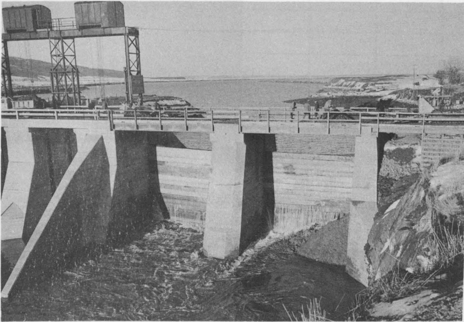
Stop logs in place in the by-pass facilities required during the construction of the Shepody River Dam. Fill is being placed on both sides of the stop logs to completely close off this structure. The permanent gate facilities on the left control the outflow of fresh water and stop the flow of tide water which previously passed up stream. March 1956.
