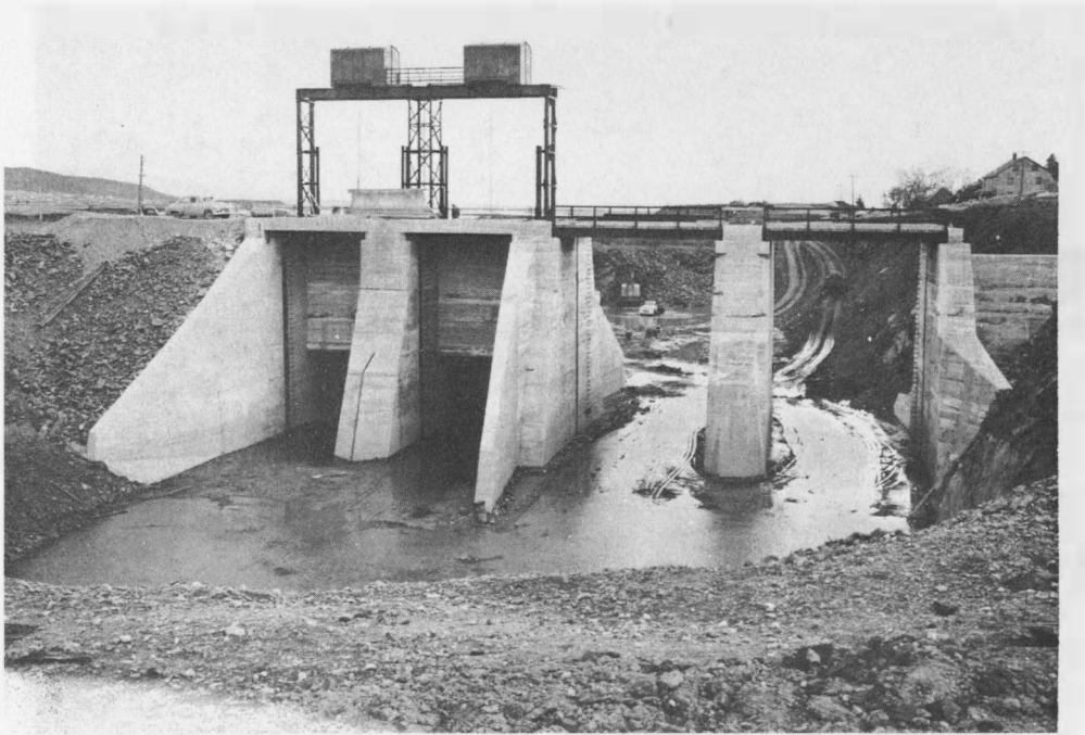
The permanent discharge gates on the left, with the temporary by-pass sluices on the right, during construction of the Shepody River Dam. The rock fill dam is to the left of the photo but closure had not yet been made pending the opening of the above by-pass facilities. When the coffer dams were removed the tidal river (rise and fall of 40 feet maximum) was partially by-passed through the above structure to permit closure of the rock fill. October 1955.
