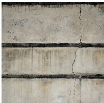
The weathering on the exterior concrete work of Brion Cemetery (Seier 2018)
