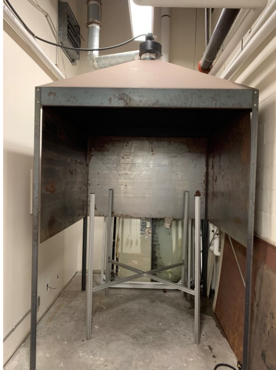
Figure 8 Smoke exhaust system with apparatus removed except for the adjustable platform framing.
