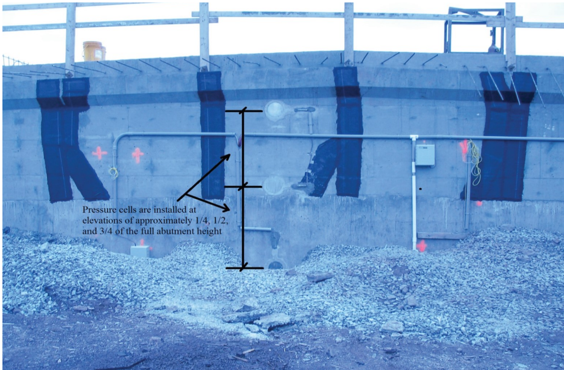
Figure 3.8: Locations of contact pressure cells installed on the west abutment. Installation locations were similar for the three contact pressure cells mounted on the east abutment (Huntley and Valsangkar 2013).
