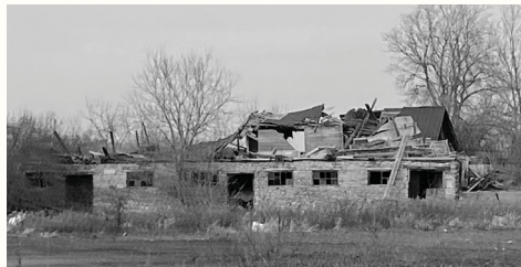
COLLAPSED BARN EAST OF TORONTO, ONTARIO 2020.
