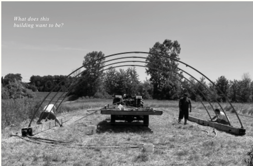
REPURPOSING GREENHOUSE FRAMES, ONTARIO 2020. WORKING WITH THE LOCAL COMMUNITY, UNUSED GREENHOUSE FRAMES FROM A LOCAL FARMER WERE RELOCATED AND REASSEMBLED TO MAKE TEMPORARY LIVING ACCOMMODATIONS.
