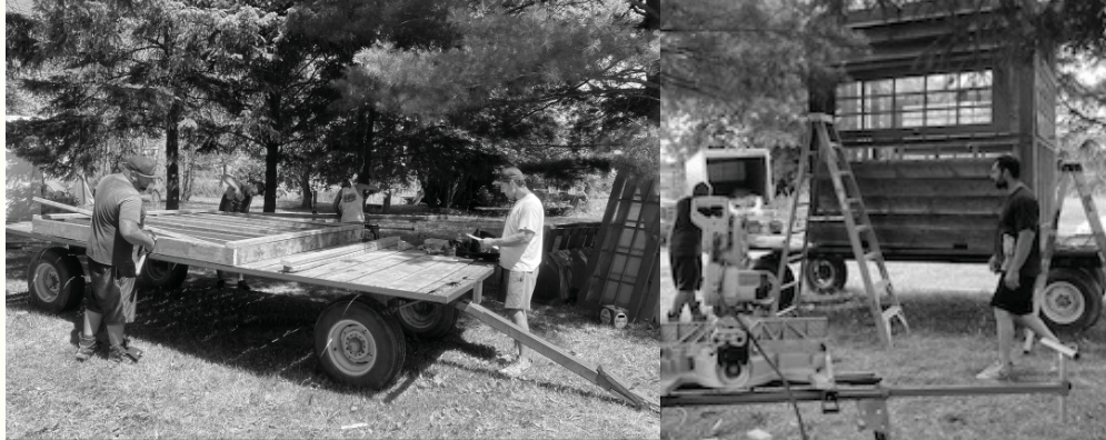
"END-OF-ROAD" MARKET STAND CONSTRUCTION, ONTARIO 2020. THE STAND WAS ASSEMBLED USING SALVAGED MATERIALS AND TESTED THE FEASIBILITY OF THE PALLETTE FOUNDATION USED IN THE THESIS DESIGN PROPOSAL OF THE SHED (see page 129).
