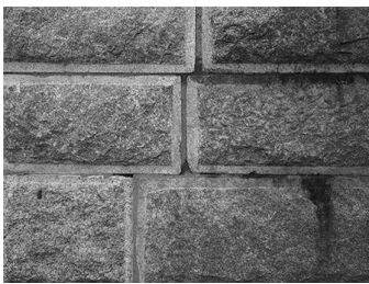
The British method of lock building used large granite blocks. These images were taken at the site of Lock 5 which was restored in 1985.
