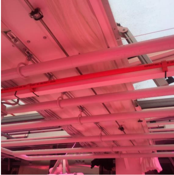
Photo 3.5: Heating and cooling pipes, production, taken by (Bashirivand, 2018)
