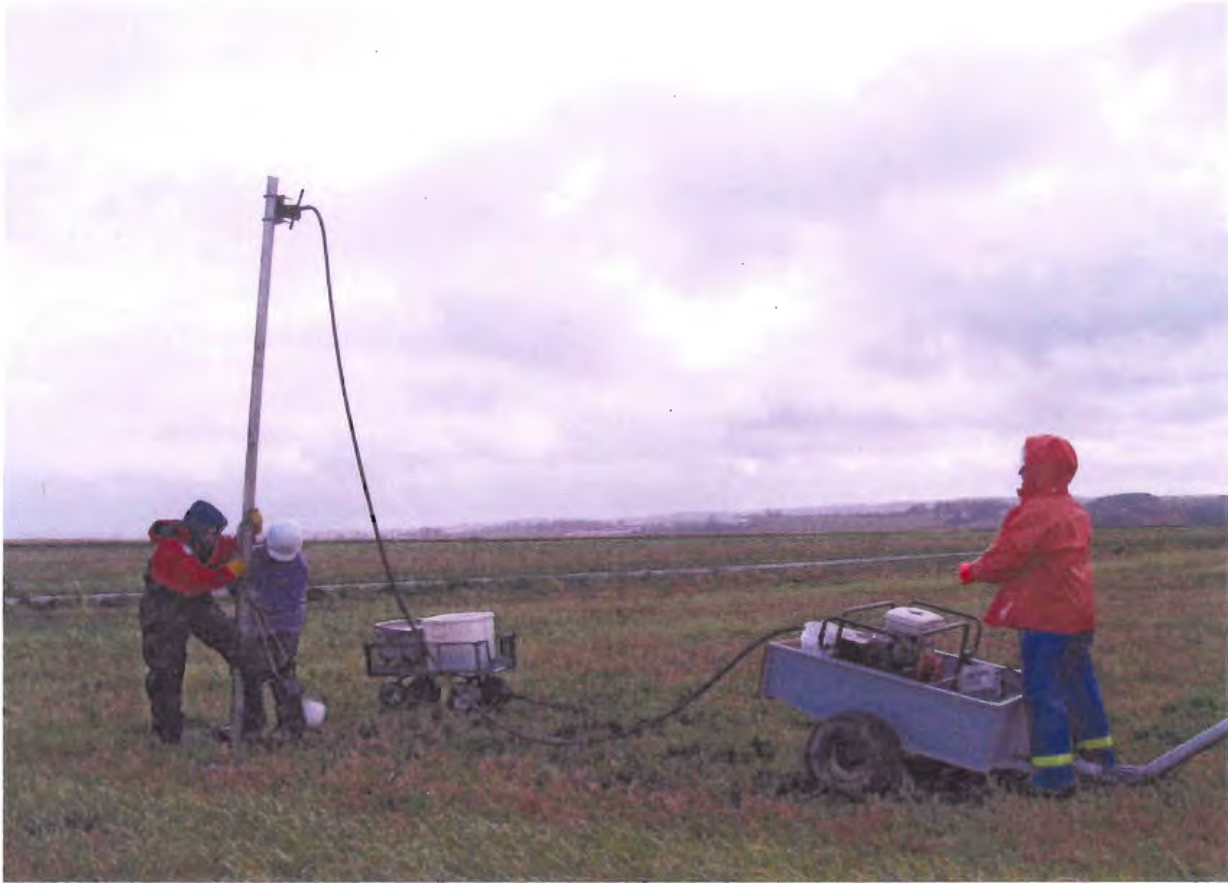
Figure 2.1: Aluminum pipe with vibrating head being vibrated into the ground at Grand Pré
