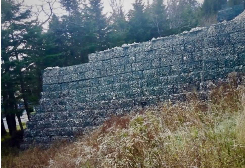
Figure 4. Retaining wall made from repurposed lobster traps in Southwest New Brunswick (Fundy North Fishermen's Association, 2018).
