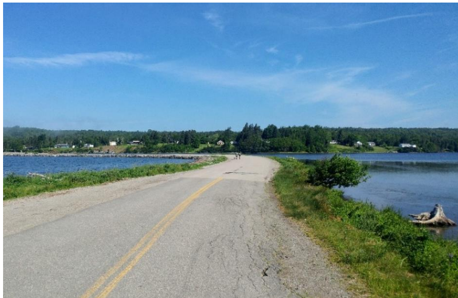
Figure 3. Chapel Rd in Cape Breton, a paved barrier decreases natural passage of water.
