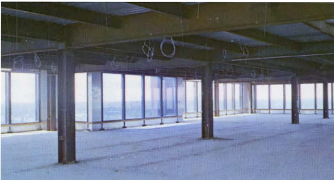
Place de Ville, Ottawa Owner: Campeau Corporation Limited Consulting Structural Engineers: John Adjeleian & Associates Ltd.
