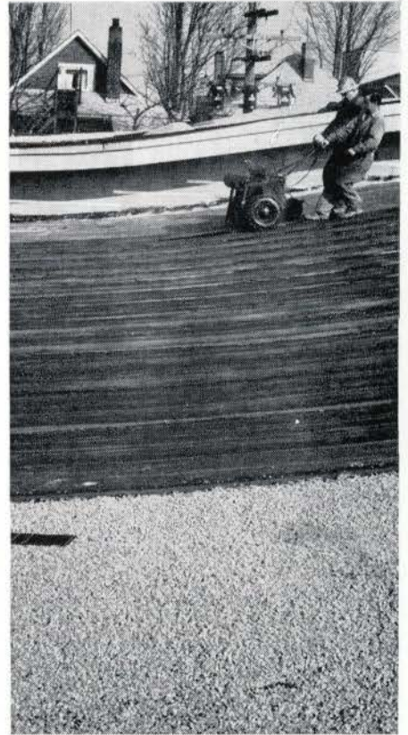
Flexible Fir Plywood panels nail easily to joists on gently curving roofs. Light weight structure utilizes 2" rigid insulation under built-up roof. Vancouver, B.C. Safeway Store. Architect - F. E. Roy.
