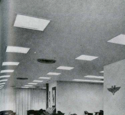
Airways Sales Office... Recessed Luminaires
