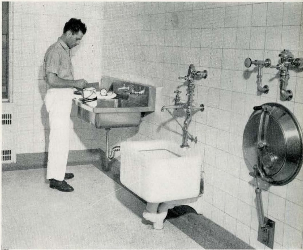
TYPICAL UTILITY ROOM
