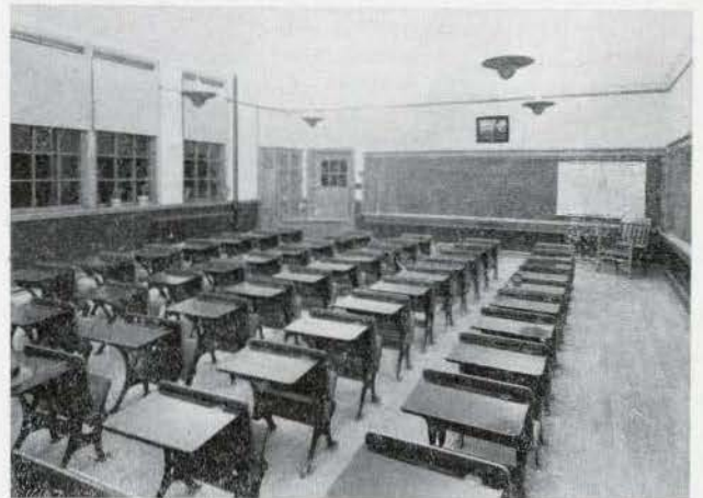
Six 500 watt totally indirect lighting units in a standard classroom.
