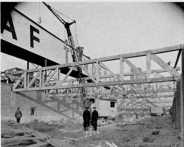
FIGURE 6 illustrates a flat Howe truss over a span of 50 feet. These trusses, it may be noted, rest on brick piers. Note truss lying on ground fully fabricated and ready for erection as a unit. This truss was designed by Gordon L. Wallace, Consulting Structural Engineer, Toronto.
