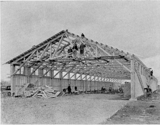
FIGURE 4 is a very good example of a mill type building. It has a triangular Pratt truss with a span of 51 feet. Note how the diagonal has been carried down to form a neat looking knee-brace. This structure was designed by T. Pringle & Son, Industrial Engineers, Montreal.
