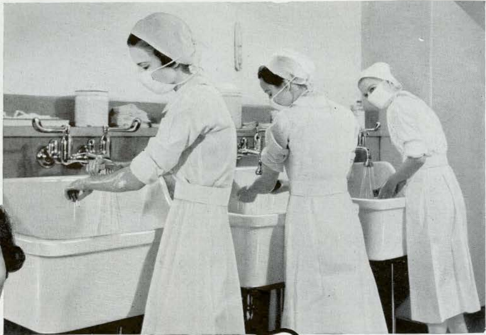
Above: Battery of Crane wash-up sinks with sprayer and wrist-action blade handles.
