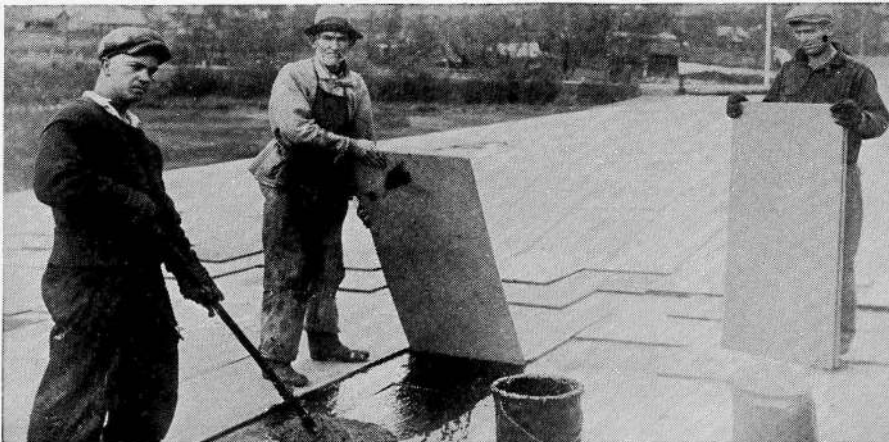
APPLYING J-M RIGID ROOFINSUL. Strong. Efficient. Especially designed for insulating roofs of industrial, commercial and institutional buildings.
