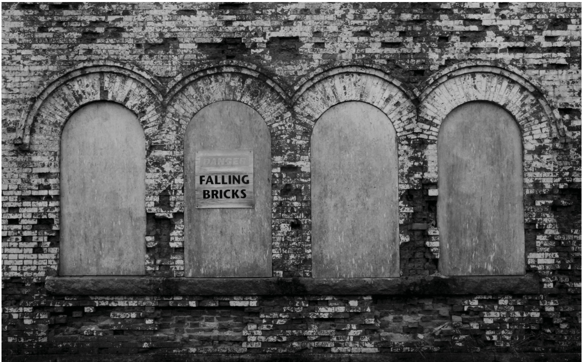
Facade of the Hazel-Hill cable station which has been closed since 1962, photograph, 2016.
