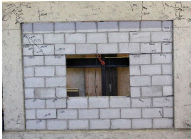
a) Overview of Infilled Frame at Failure
