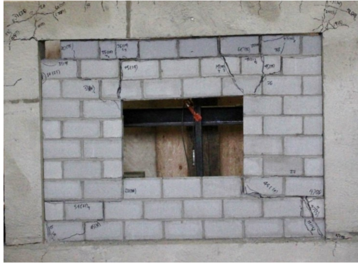
a) Overview of Infilled Frame at Failure
