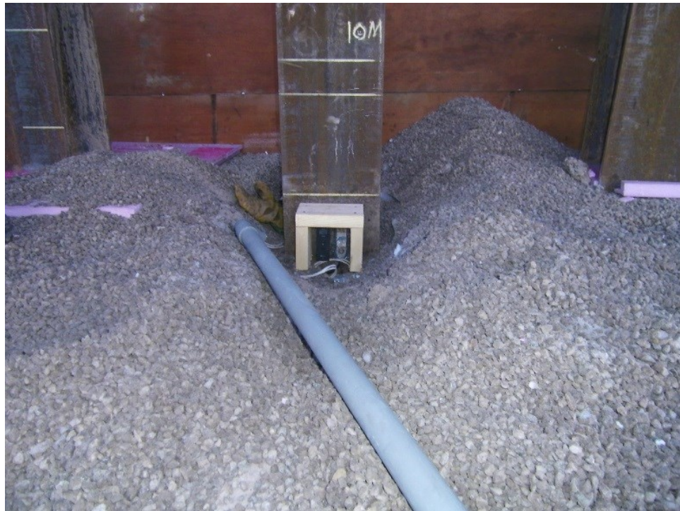
Figure 3.15 Strain Gauges and Wireless Thermometer Installed on Pile P5N.
