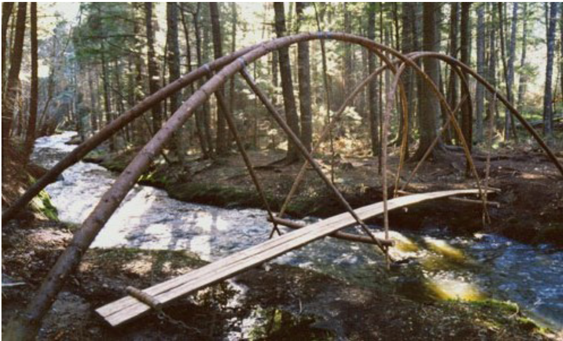
Bartel Bridge: Richard Kroeker & Alvin Bartell, part of thesis project at the TUNS.
