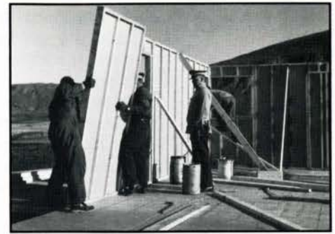
Figure 17. Mounted Police detachment building under construction at Alexandra Fiord, Ellesmere Island, 1953. Consisting of lightweight, prefabricated plywood components, the building could be quickly erected with little difficulty. (National Archives of Canada, PA 176634)
