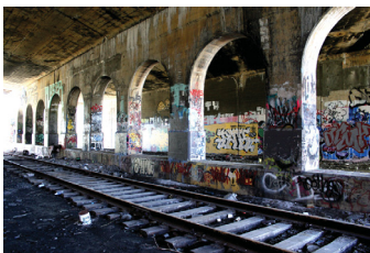
Bridge in Dequindre Railway Cut prior to transformation into greenway. (Jeff O'Brian, 2006)
