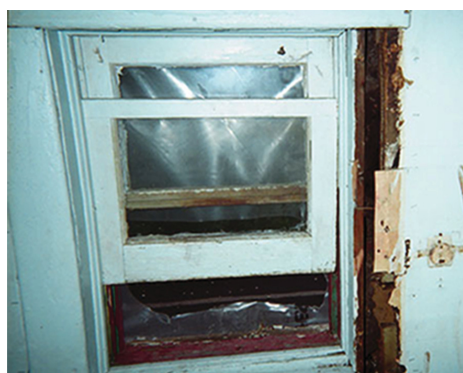
Substandard housing, photo-voice project, PHM, Laurentian University
