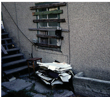
Substandard housing, photo-voice project, PHM, Laurentian University
