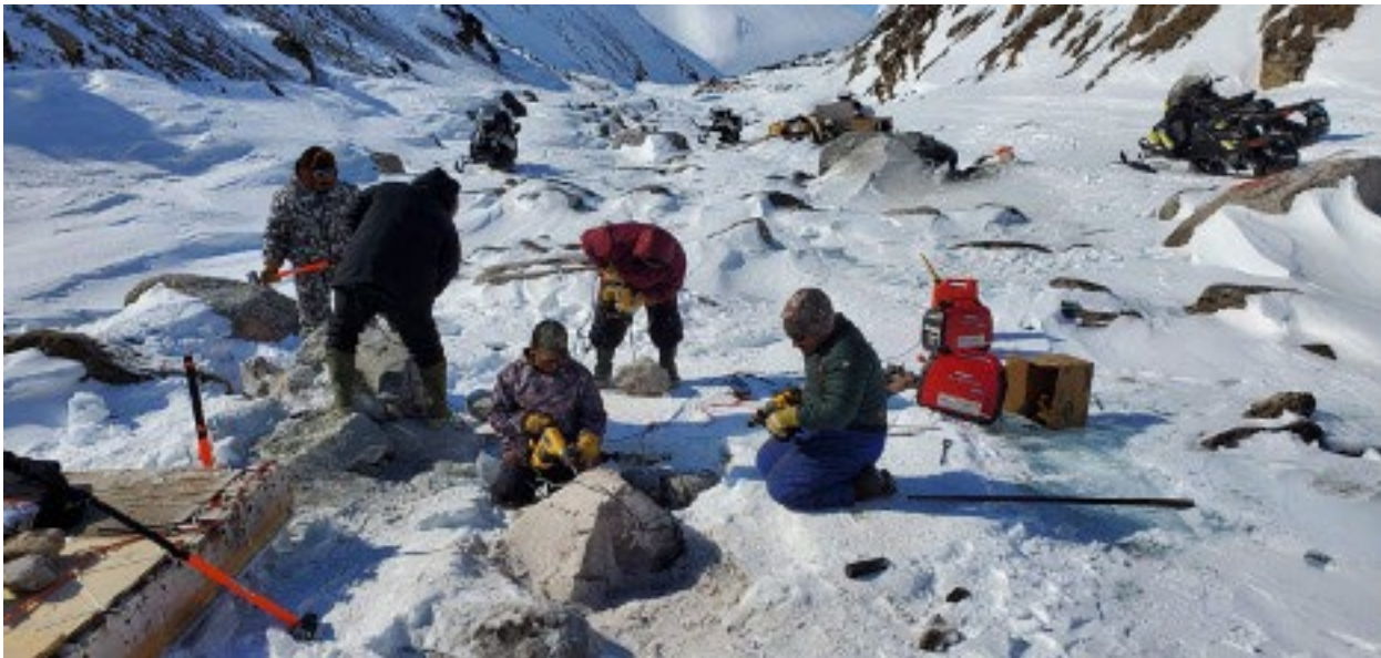
Figure 16. Community members clearing rockfall on Canyon River
