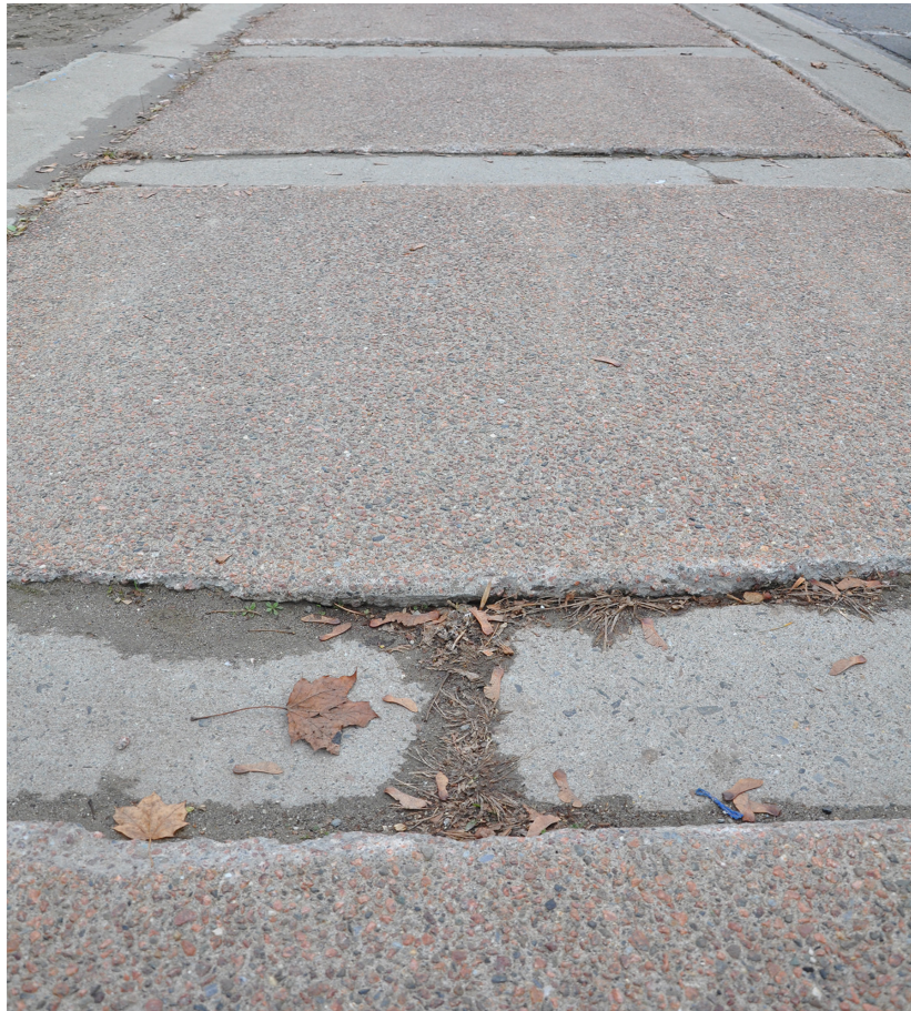
Figure 38. Frost Heave and Cracking sidewalk surfaces. St. Stephen NB. Hazardous Circulation routes for our seniors
